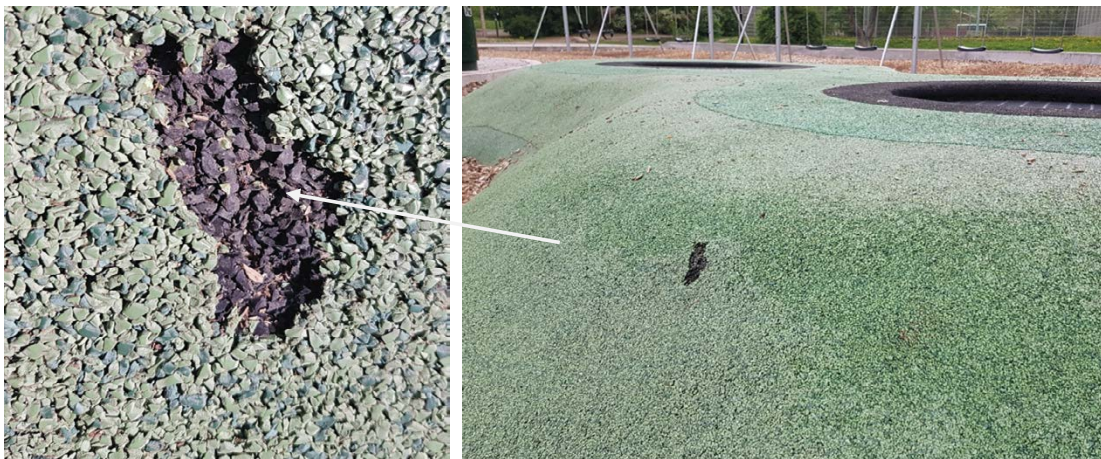
Figure 3. Fall safety surface where the top layer has been damaged and the base layer is exposed. Photo: Åsa Jarsèn.
