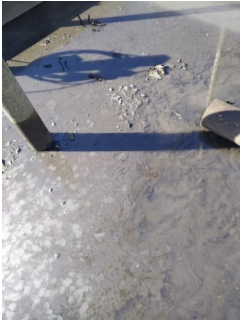
Figur 18 Sediment i R1 under renovering GC-tunnel.
