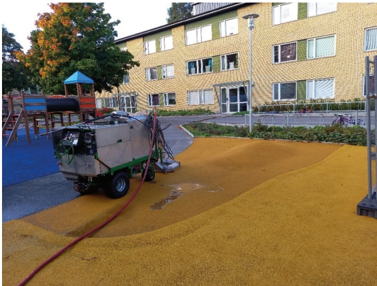
Figure 39. Photos taken after cleaning.
