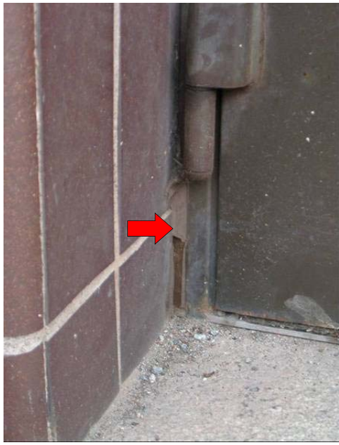
Sealant adjacent to steel door
