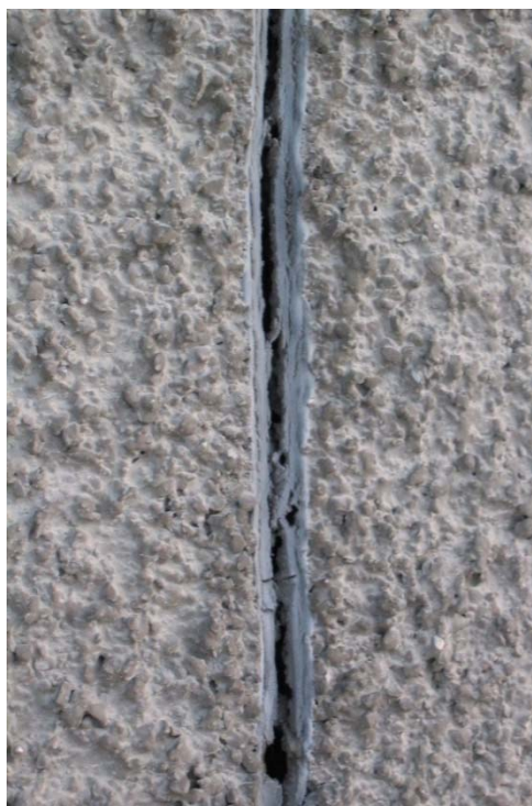
Cracked sealant between concrete facade elements
